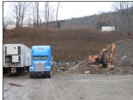
View of failure 1 from Harold Neale Excavating Company
