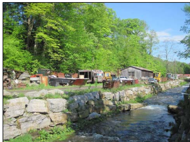
Rock cross vane grade control structures extending from the Ogden Street bridge to station 32+50
