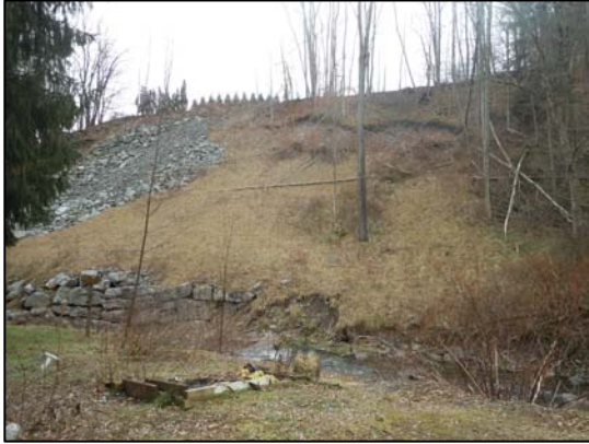
View of failure 2 from opposite side of brook
