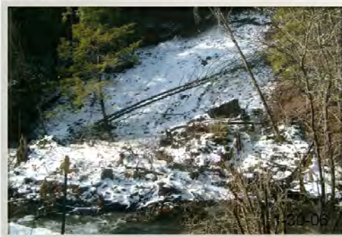
Erosion – Mass failures
