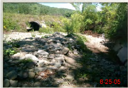
Deposition – Undersized Hydraulic Structure
