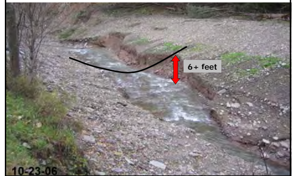
This slope was actively migrating as the stream continued to lower its bed to adjust its profile. This increased potential risk to those downstream.
