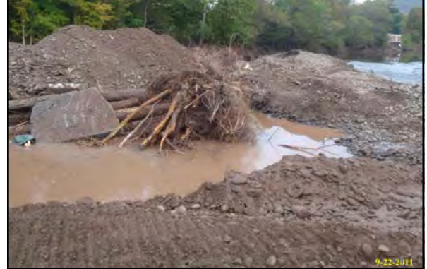
Root wads were placed in two layers with large rocks to hold them in place.
