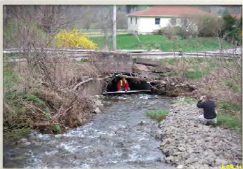
Deposition – Undersized Hydraulic Structure
