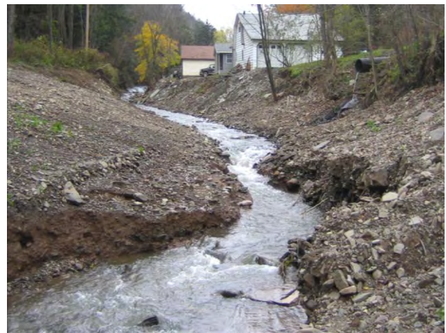
Figure 2.16 Headcut on Third Brook stream in Walton, NY
