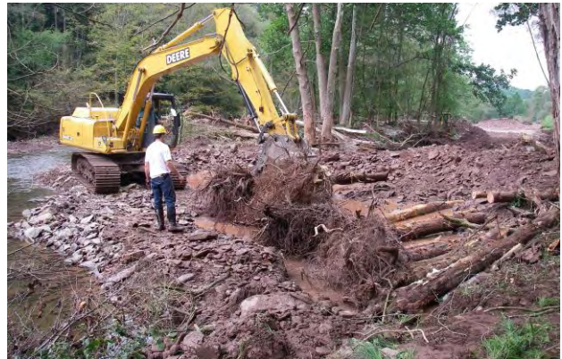
Root wads were placed in two layers with large boulders or logs to hold them in place
