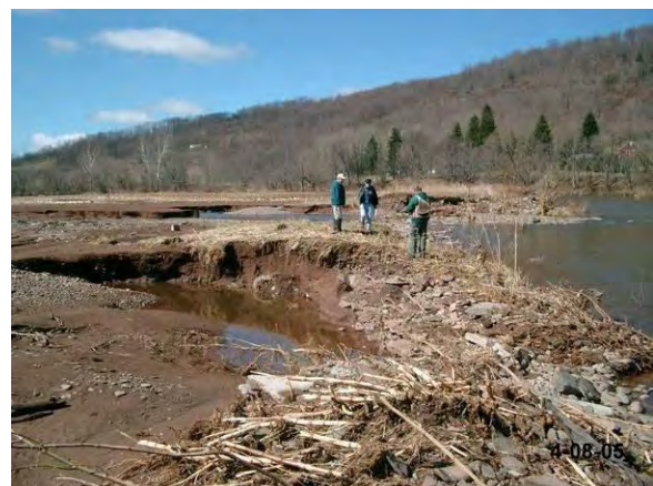
Figure 3.11 Berm that was breached in 2005 storm event
