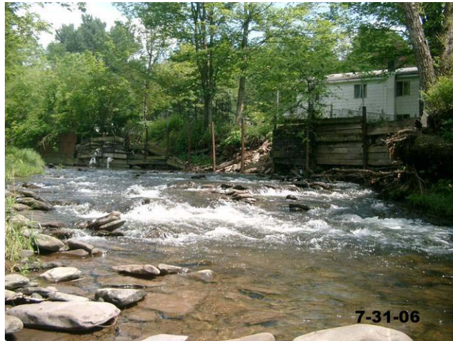
Figure 1.8 Failing Revetment Wall
