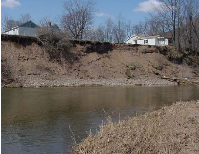
Figure 7.6.6 Looking at a high eroding bank on the left side at Terrace Avenue potential project site.
