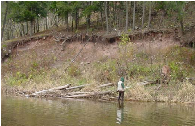
Figure 7.4.2 High eroding right bank located approximately 2,600 feet upstream from County Bridge 33.
