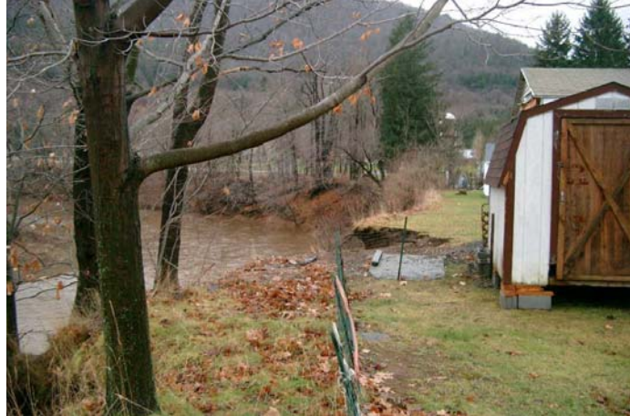
Figure 2.6 View of relocated shed along severely eroding bank at the Terrace Avenue site. Note area near center of photo where upstream edge of shed was located (December, 2004).
