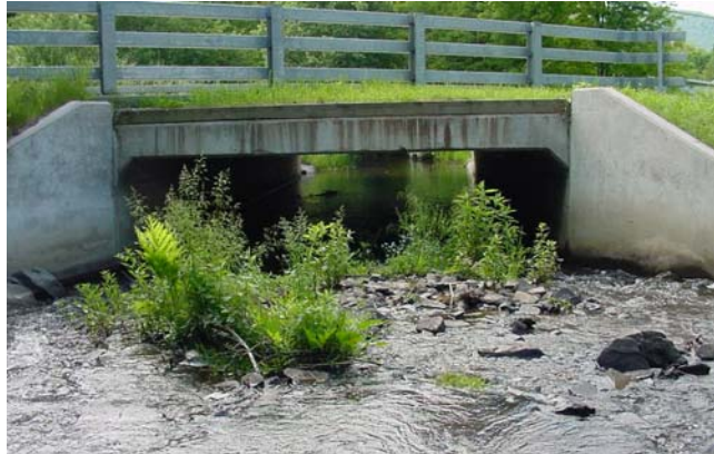
Figure 7.2.3 Deposition at the upstream end of the box culvert located on River Street.
