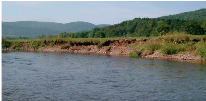
Figure 7.5.1 Typical eroding bank along agricultural field with no riparian buffer approximately 4,000 feet downstream of Platner Brook.
