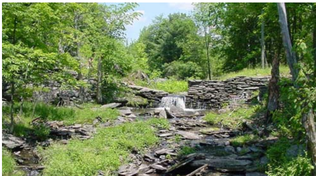
Figure 7.2.2 Remains of the old mill dam located approximately 375 feet upstream from River Street stone arch bridge.
