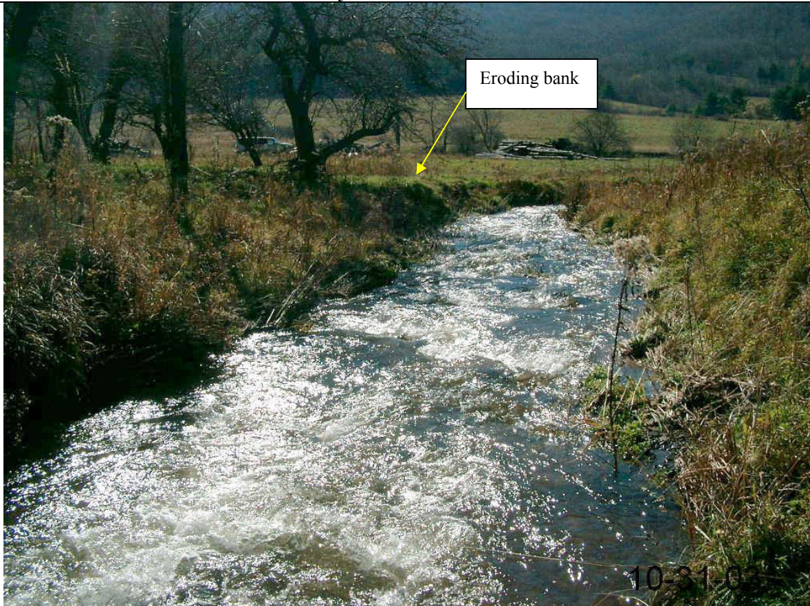
Photo 6.17: Just below culvert, 10-31-03. Stream entrenched with no floodplain.
