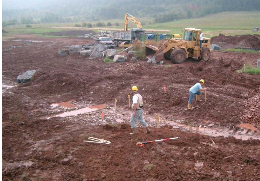
Figure 6.16 Photo taken during construction showing newly excavated channel and layout for a vane structure.
