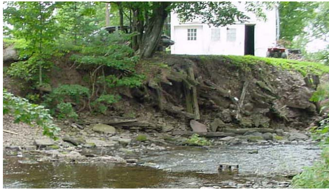
Figure 7.3.13 Looking downstream at an eroding bank located approximately 1,750 feet upstream from County Bridge 18-6.
