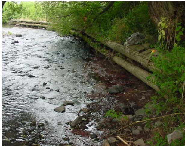
Figure 7.3.8 Log cribwall on the right bank located approximately 1,200 feet downstream from Town Brook confluence.
