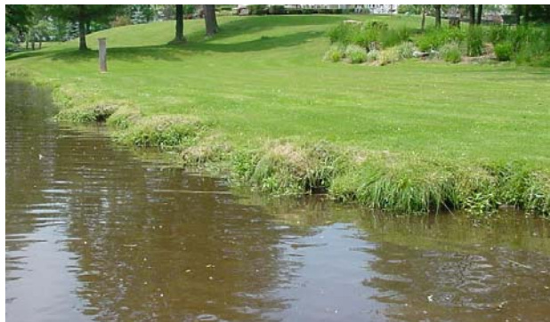
Figure 7.2.6 Lawn maintained to edge of water located approximately 350 feet upstream from Railroad Avenue culvert.
